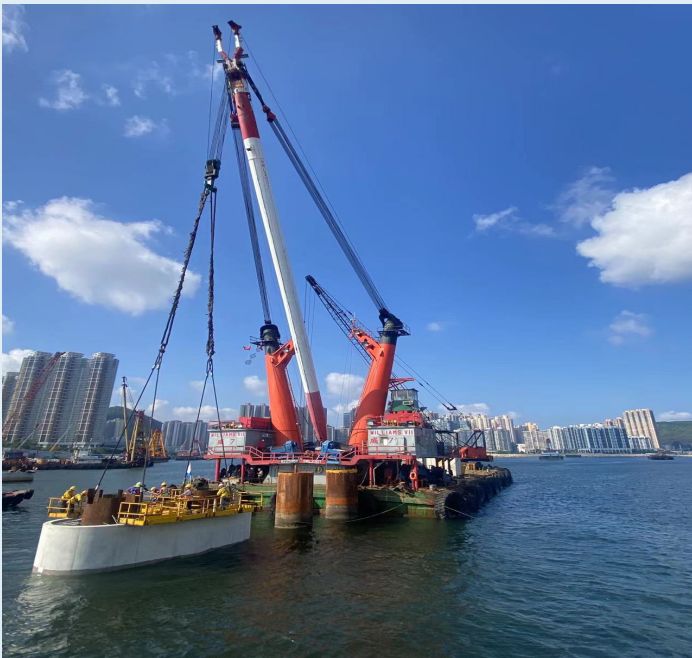
香港将军澳大桥吊装水下桥墩 Lifting Installation of Underwater Piers of Tseung Kwan O Bridge, HK
