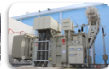
220kV/110kV GIS Binh Tan Hochiminh (2008)
