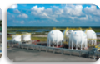
Ca Mau gas processing plant Ca Mau, Vietnam
