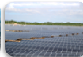
Ninh Phuoc plant, 50MW Vietnam (2019)
