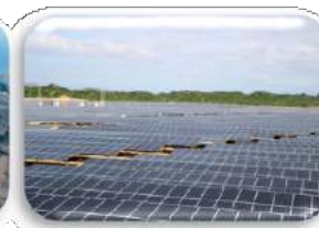
Ninh Phuoc plant, 50MW Vietnam (2019)
