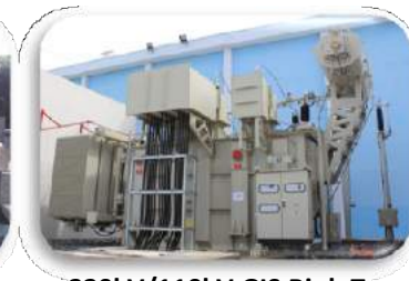
220kV/110kV GIS Binh Tan Hochiminh (2008)
