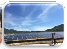
Cam Lam plant, 50MW Vietnam (2019)
