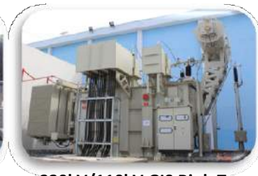
220kV/110kV GIS Binh Tan Hochiminh (2008)
