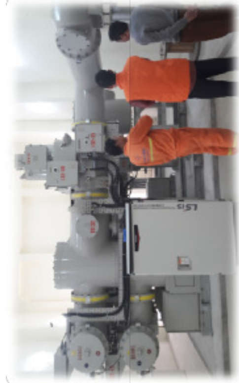
110kV GIS Vinh Yen 2 substation (2015) Trạm 110kV GIS Vĩnh Yên 2 (2015)
