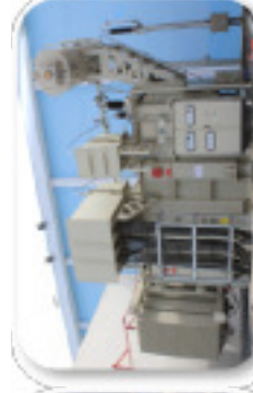
220kV/110kV GIS Binh Tan Hochiminh (2008)
