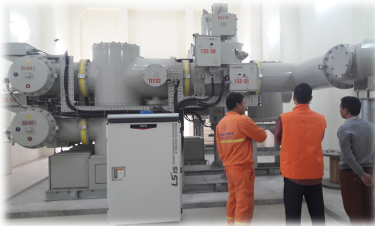
110kV GIS Vĩnh Yên 2 substation (2015) Trạm 110kV GIS Vĩnh Yên 2 (2015)
