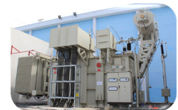
220kV/110kV GIS Binh Tan Hochiminh (2008)
