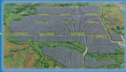
Thanh Long Phu Yen Solar Power Plant (50MWp)
